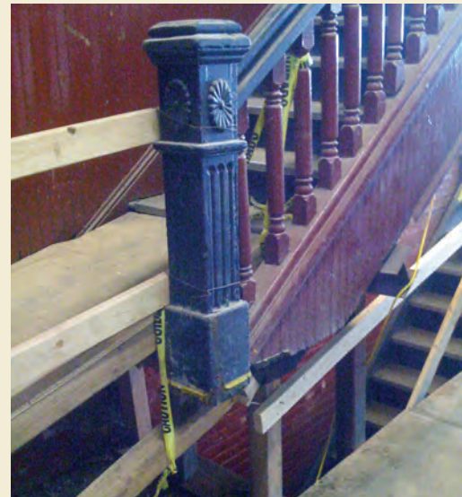
Historic preservation provides the opportunity to save beloved building elements that show the public that we believe in preserving the department’s institutional heritage.
