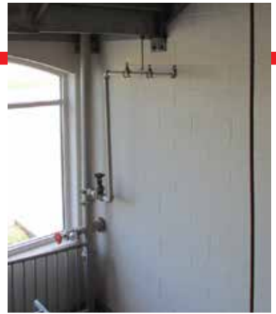
A dry standpipe and sprinkler training prop in training stair/tower.
