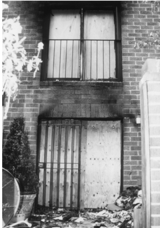
Photo 3 Sliding glass doors and security bars as viewed from inside the patio fence.
